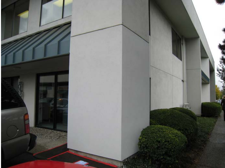
Description: Finish coat applied with texture and color matched to existing building color.
