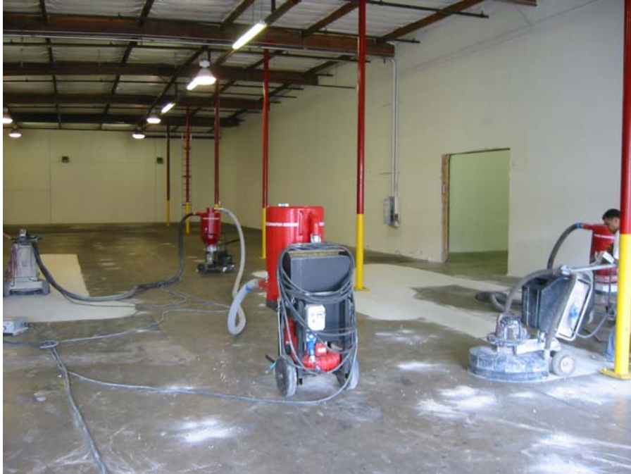
Description: Warehouse Floor. Start of diamond grinding. The difference is immediately noticeable.
