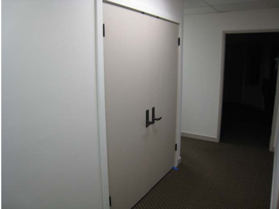
Description: New server room doors with matching mortise hardware blanks.
