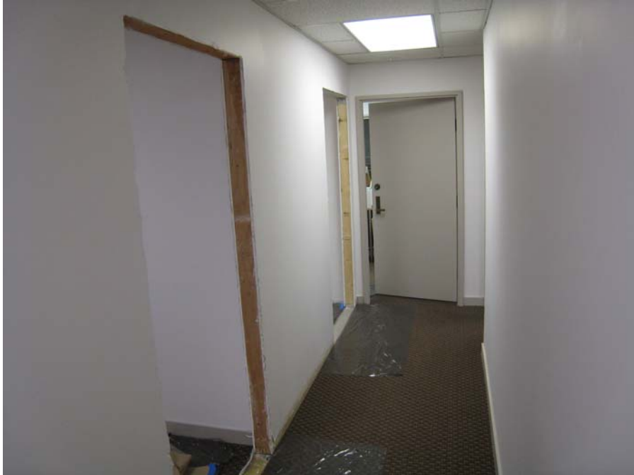
Description: Partition walls installed for new offices and doorways cut into hallway for access ready for doors.
