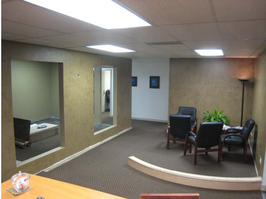
Description: Wall demolished and rebuilt ready for glass block paneling. Curved Red Oak reception desk curb installed.
