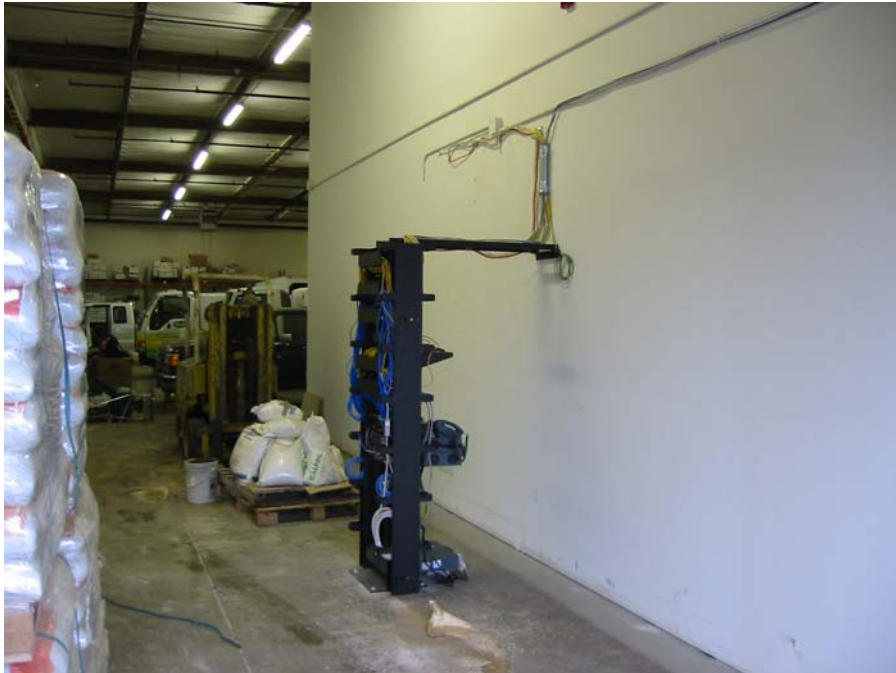
Description: Existing condition. Server rack mounted to the floor, powered by an extension cord through the wall.
