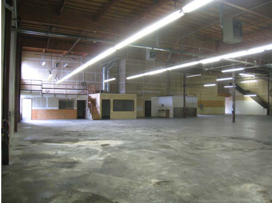
Description: Existing warehouse condition with drop lighting and dual 4" electrical gutter runs.
