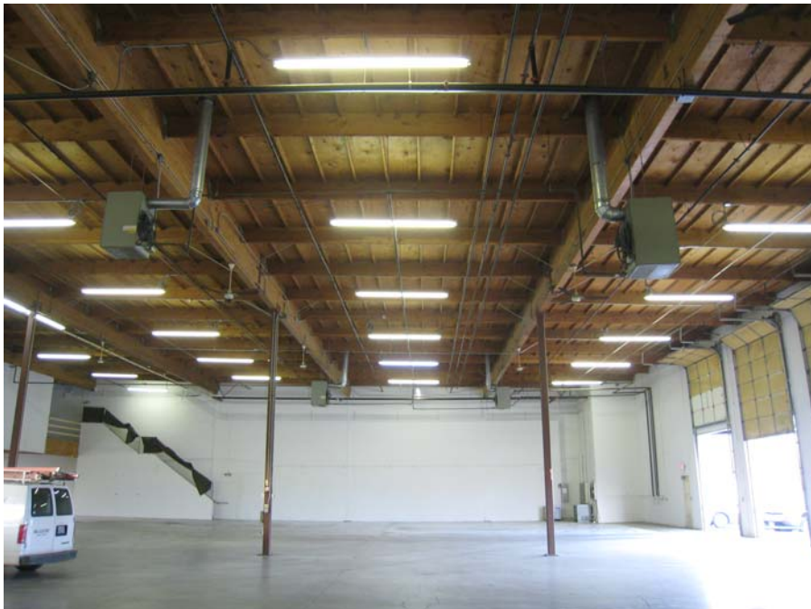
Description: Warehouse lighting re-balancing into clean “rows”.
