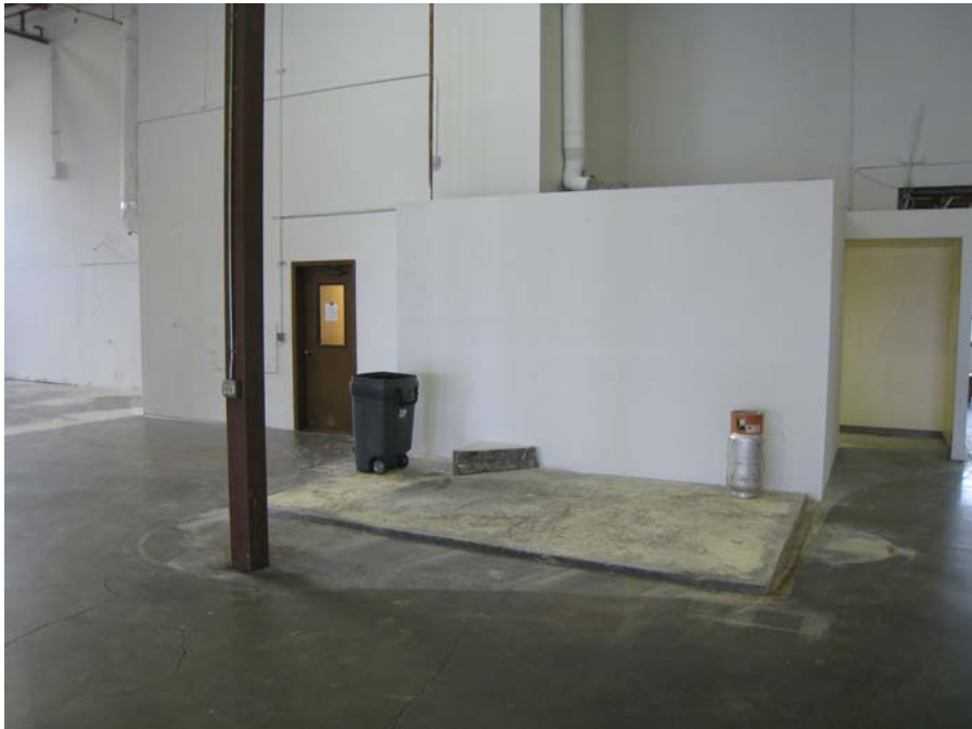
Description: Wash area completed, cleaned and re-drywalled the face from moisture damage and painted.
